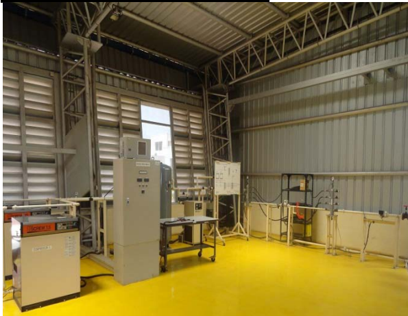
Compressed Air System Lab
