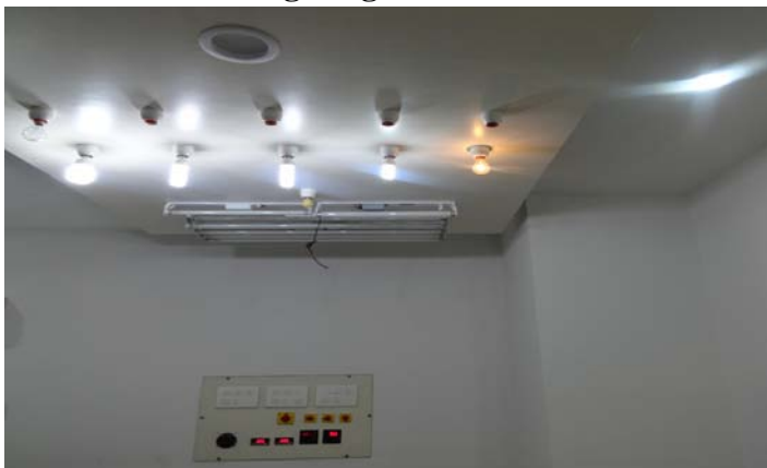
Indoor Lighting Lab
